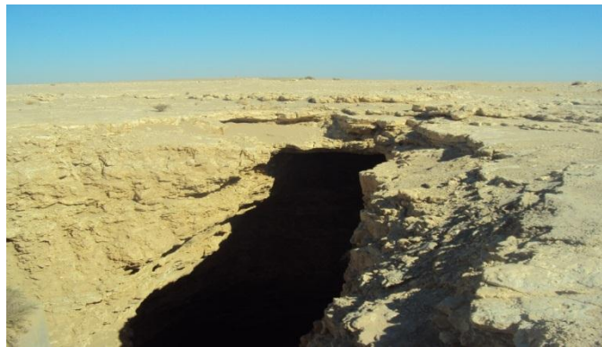
Lacks and cracks in Umm Dahl well
